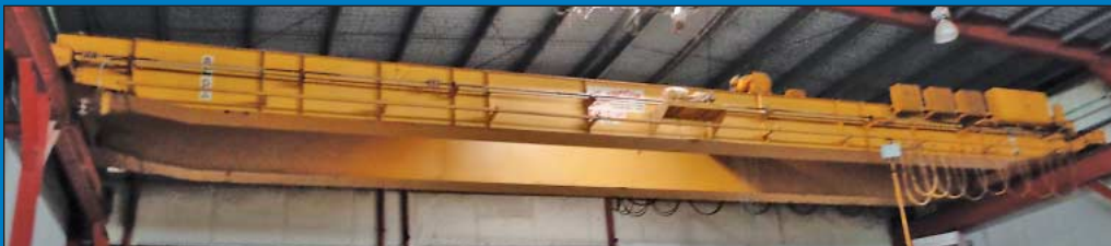
10 Ton X 57' Span (Approx.) Konecranes Double Girder Top Running Overhead Crane
