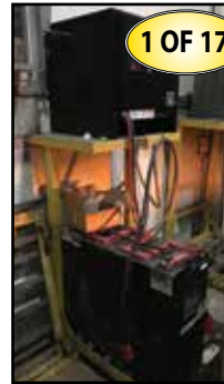
(17) 36-Volt Battery Chargers
