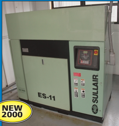
NEW 2000 50 HP Sullair Model ES11-50H Cabinet Enclosed Rotary Screw Air Compressor
