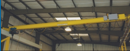
3 Ton X 35' Approx. Span X 85' Approx. Long North American Industries Free Standing Overhead Bridge Crane System
