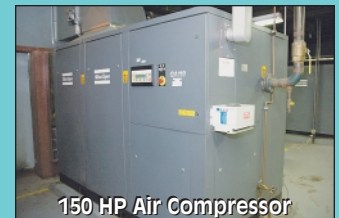
150 HP Air Compressor
