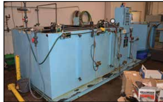
MASTER CHEMICAL Coolant Filtration System
