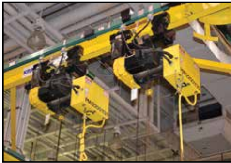
Approx. 40' x 60' Overhead Monorail System
