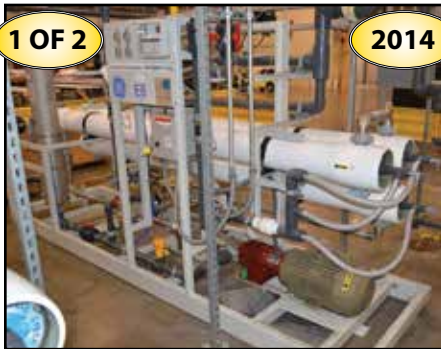
(2) 2014 GE NC Reverse Osmosis Systems
