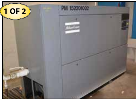
(2) ATLAS COPCO 75-HP Air Compressors
