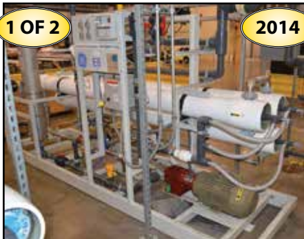
(2) 2014 GE NC Reverse Osmosis Systems
