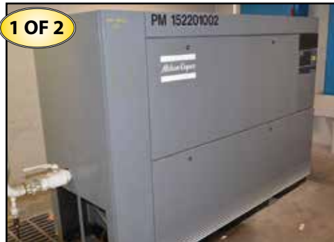
(2) ATLAS COPCO 75-HP Air Compressors
