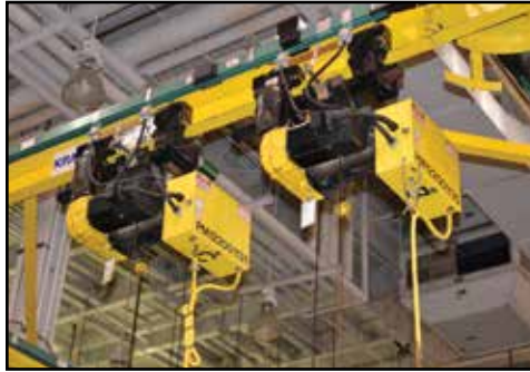
Approx. 40' x 60' Overhead Monorail System
