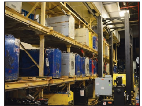
(42) 24-VOLT TO 48-VOLT BATTERIES
