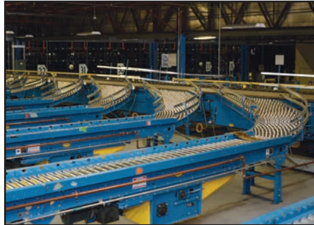
2,000+/- HYTROL 15' MULTI-LANE POWER ROLLER CONVEYOR
