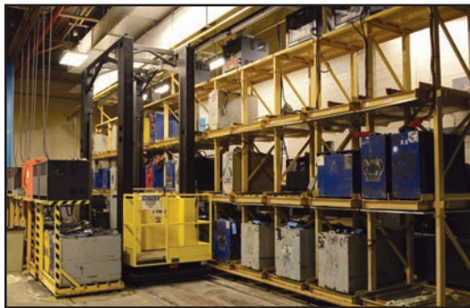
MTC BATTERY STORAGE & RETRIEVAL SYSTEM
