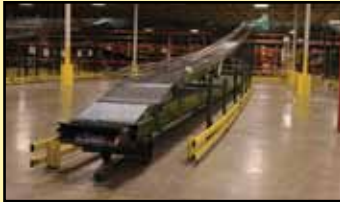
Approx. (20) RAPISTAN DEMATIC Trailer Loader Conveyors
