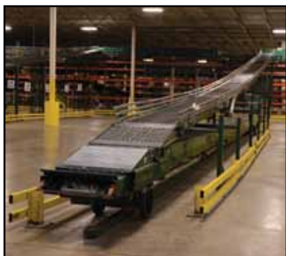
Approx. (20) RAPISTAN DEMATIC Trailer Loader Conveyors
