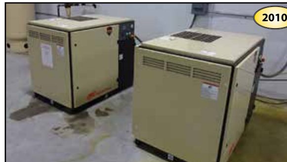
(2) 2010 INGERSOLL RAND SSR UPG-30-125 30-HP Air Compressors
