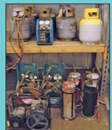
Partial View Refrigeration Equipment
