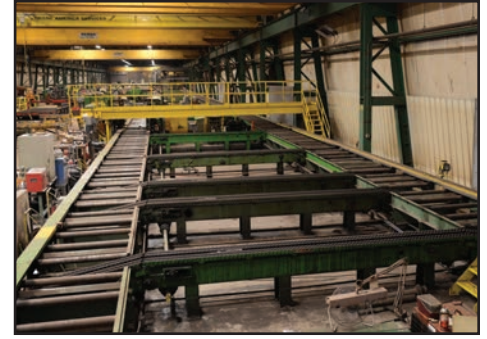
POWER ROLLER CONVEYOR LINES
