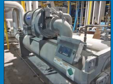
**Carrier Model 19XR-2022294BHS64 Centrifugal Chiller
