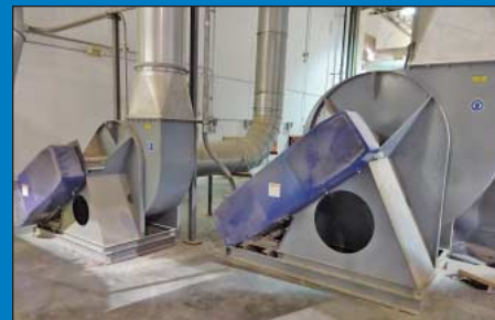
125 HP, 75 HP, 60 HP, & 30 HP Disa Blowers
