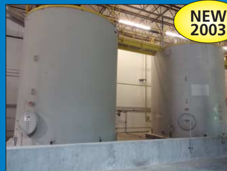
(4) 20,000 Gal. Mild Steel Bulk Storage Tanks
