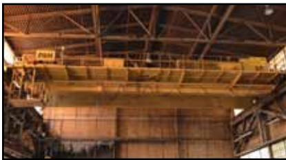
(2) P&H 45/15 Ton Twin Girder Bridge Cranes
