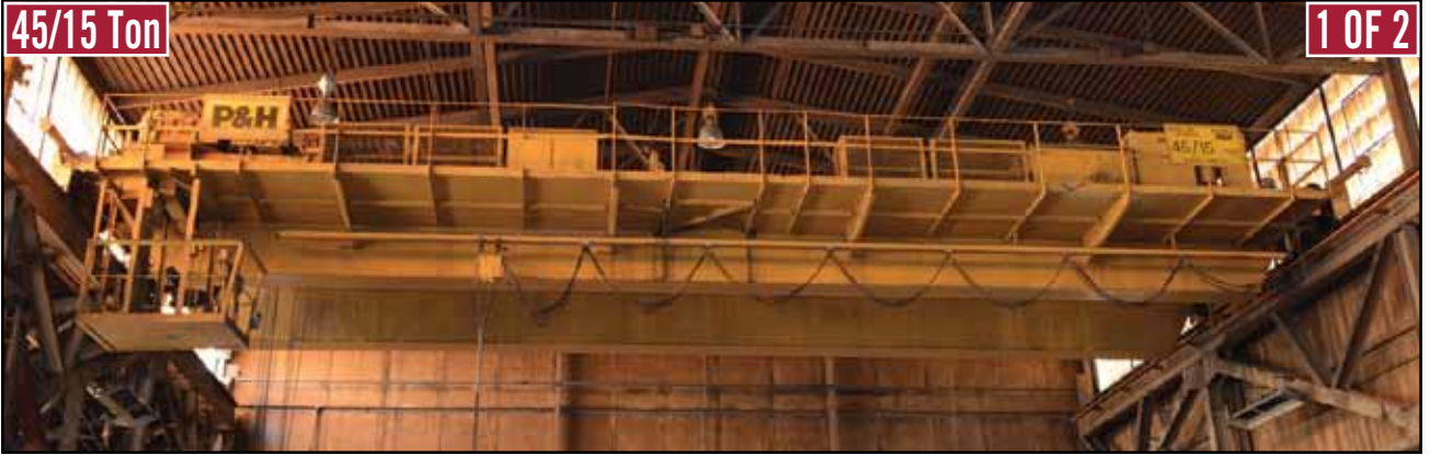
(2) P&H 45/15 Ton Twin Girder Bridge Cranes
