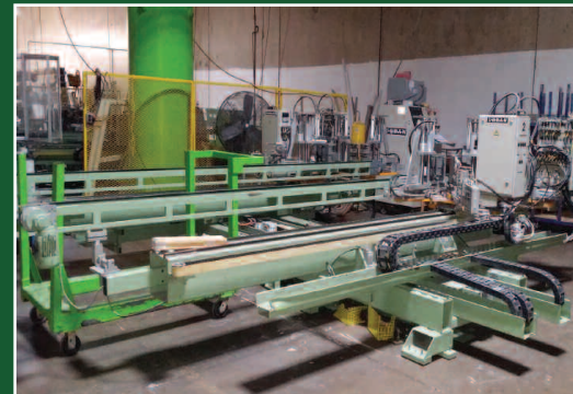
View of the Glass Tempering Line
