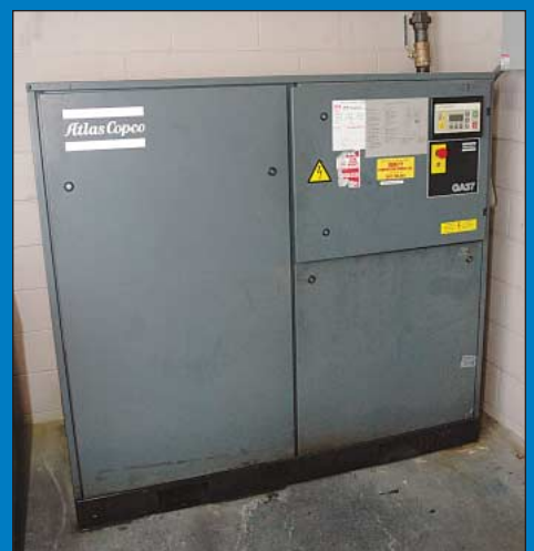
50 HP Atlas Copco Model GA-37 Cabinet Type Rotary Screw Air Compressor
