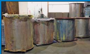
Partial View Stainless Steel Tanks
