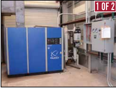
1 of 2 QUINCY QSI-500 Rotary Screw Type Air Compressors
