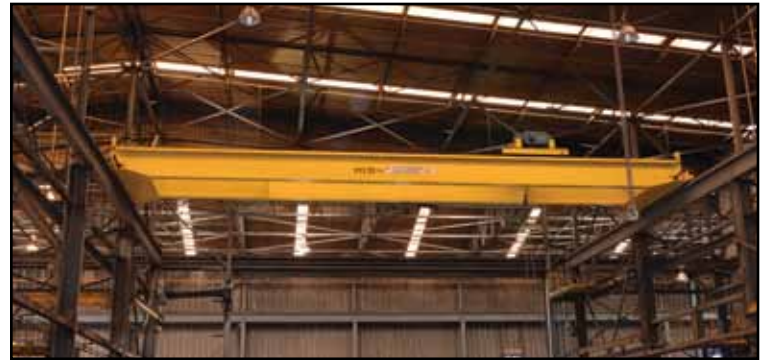
NORTH AMERICAN 20-Ton Bridge Crane
