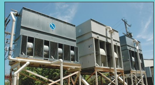
Bank View (3) BAC Cooling Towers
