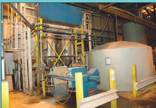
Overall View Waste Water Treatment System Including JWI Filter Press
