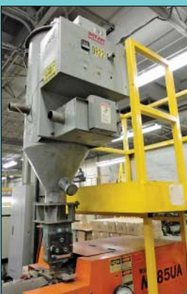
(10) Bry-Air Model RD-50 Dehumidifying Dryers Including Some w/ Hoppers
