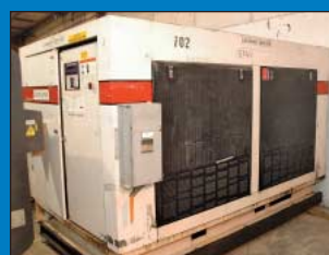
200 HP Gardner Denver Model EDPSA Cabinet Enclosed Rotary Screw Air Compressor
