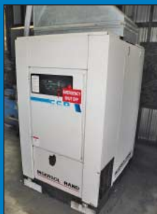
50 HP Ingersoll Rand Model SSR-EP-50SE Rotary Screw Cabinet Type Air Compressor
