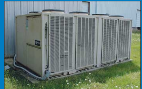
Trane Model CGACC804RANJJ40GM Central Chiller Unit
