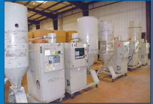
Partial View (2 of 7) Conair Dehumidifying Dryers w/ Hoppers
