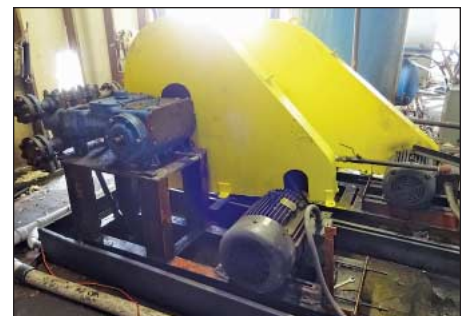
(2) 25-HP High Pressure Pumps
