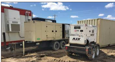
183 KVA Doosan / Ingersoll Rand Model G185 Diesel Powered Generator
