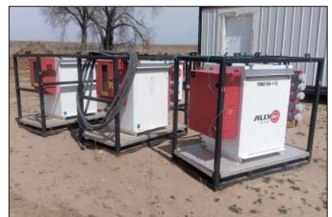
(7) 150 KVA Trystar Portable Power Distribution Units
