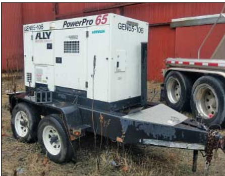
(2) 63 KVA Airman Model Power Pro65 Diesel Powered Portable Generator
